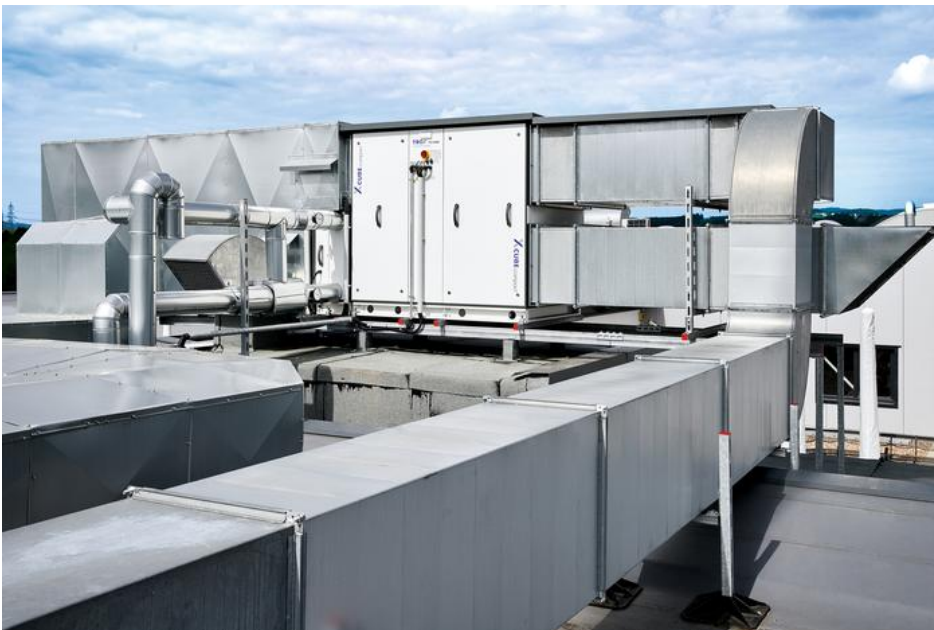
X-CUBE compact air handling unit on the roof of Werthmann workshops in Attendorn, Germany.
